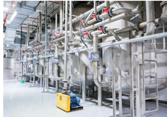
Performing filtration system designed by ANDRITZ
